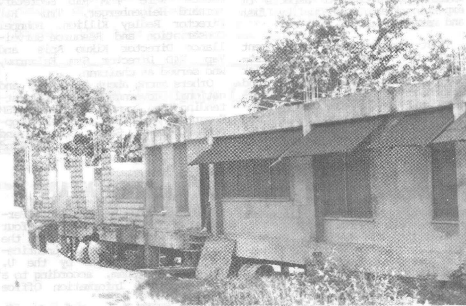
INCOMPLETE CCM DORMITORY - FSM Public Auditor John Dye said in a Nov. 16 report that the Community College of Micronesia administration is ultimately responsible for management of funds for construction of the new CCM dorm which started in 1981 and is incomplete "despite expenditures of at least $303,457." The original bid was $157,732 for the construction. This is a Nov. 27 photo of the dorm.
