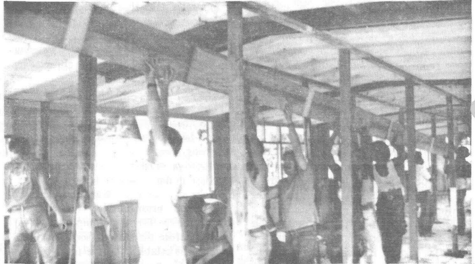
REPLACING CEILING BEAM--PATS students and instructors and Peace Corps volunteers are replacing the ceiling beam in the former Navy bachelor officers' quarters in Kolonia as part of the renovation of the state-owned building to be used as the Micronesian Legal Services Corp. office in Ponape. (Photo by Jack Petry)
